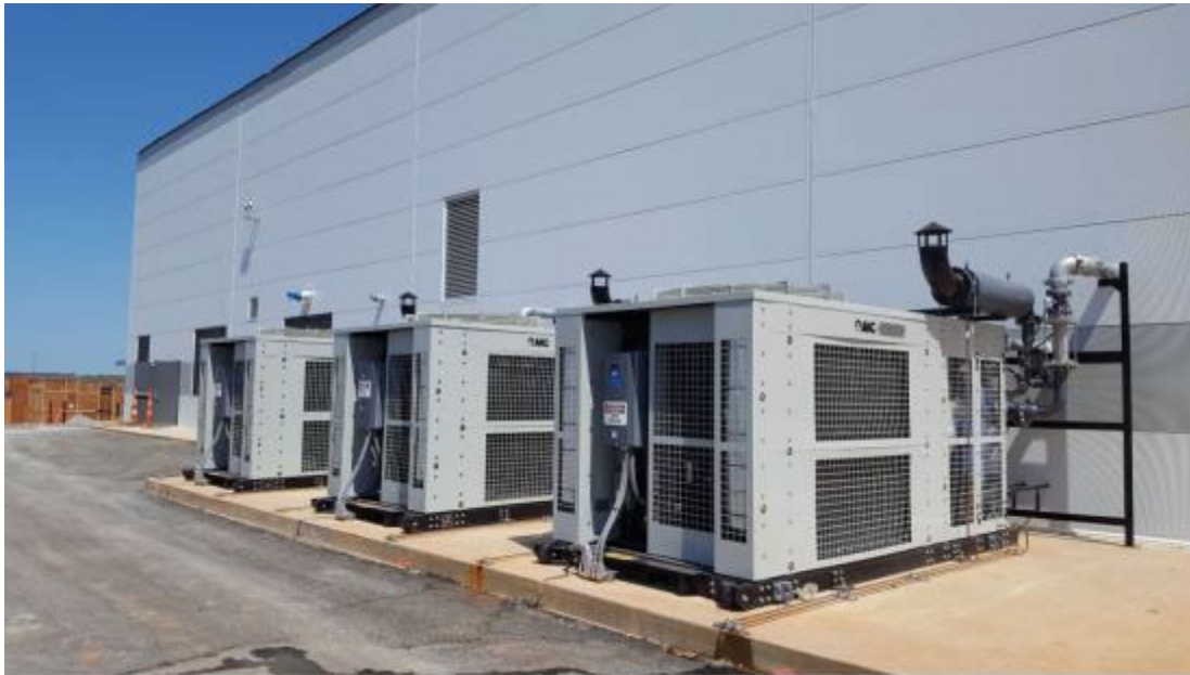
Air cooler skids for centrifugal air compressors.
