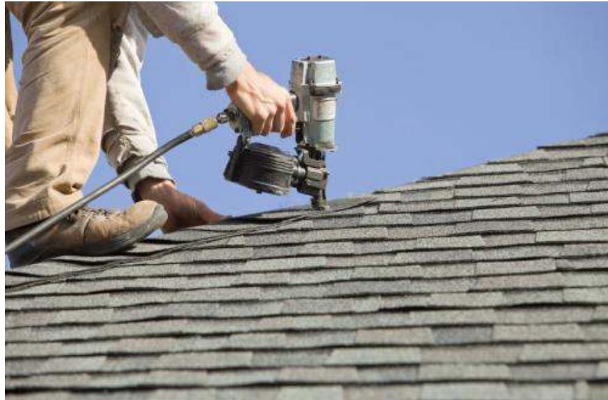
Rofer using an efficient pneumatic nail gun operating from a small gasoline powered or electric powered air compressor.
